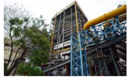
View of Boiler, Vijayanagar
